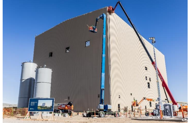
도표 3. Sodium Test and Fill Facility(1)
